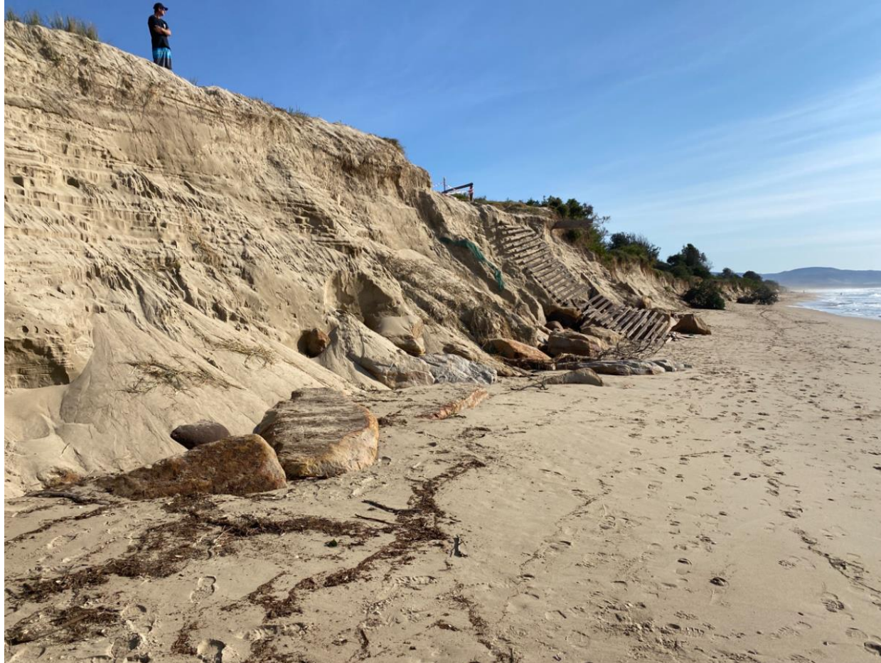
Figure 11. Shoalhaven Heads Surf Club dune following August 2021 event with part of historic rock revetment visible (source: Shoalhaven City Council Coastal Monitoring Viewer)
